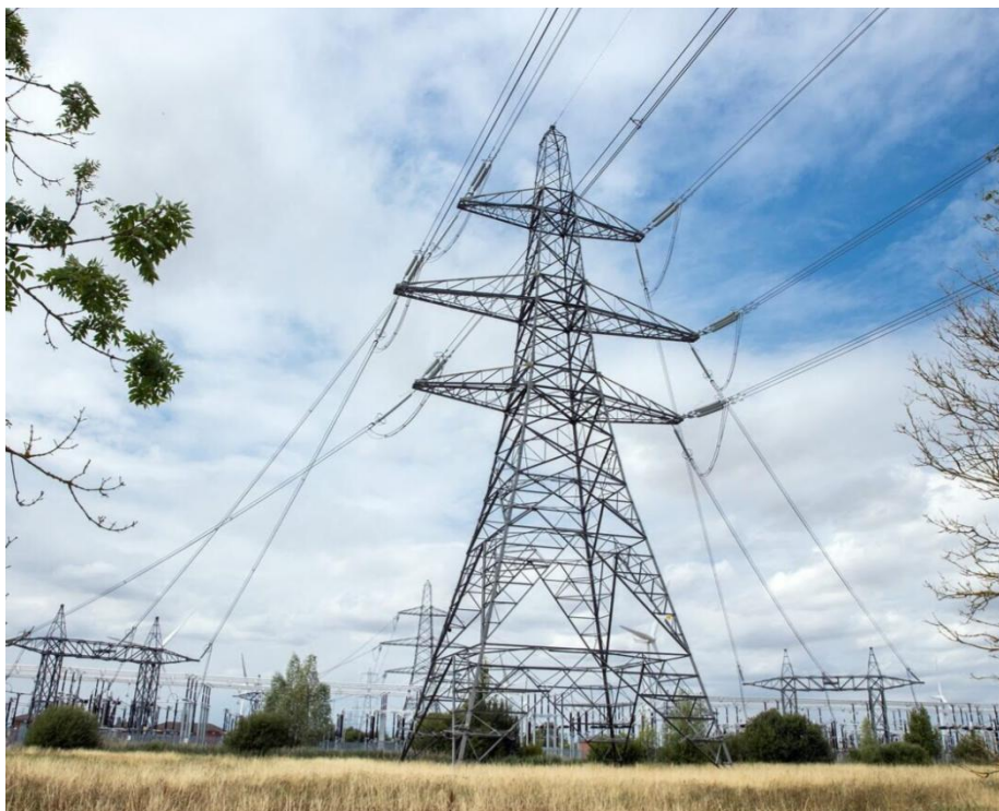
Image 5.13 Typical terminal lattice pylon 3
